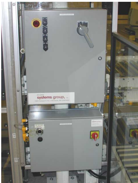
Honeywell SDS interface to I/O devices
