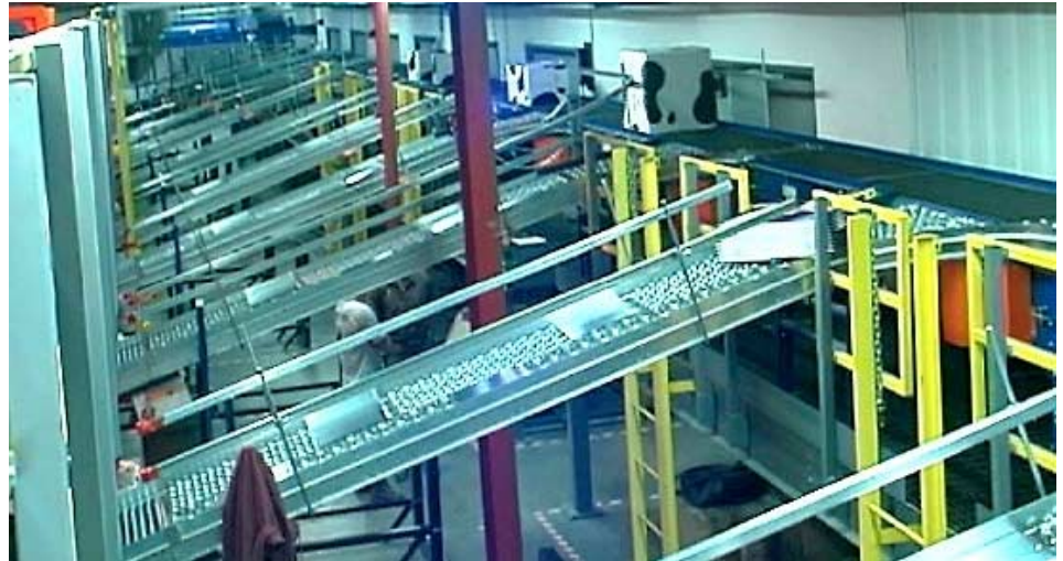
Gateway’s North Sioux City auto-sort material handling system — downramps ( center) deliver cartons to trailers through the dock doors (left)
